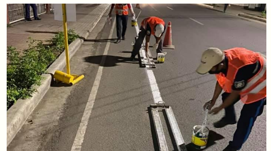
The Traffic Enforcement Agency of Mandaue (TEAM) personnel worked overtime to install bike lanes along A. Del Rosario St., Barangay Guizo, Mandaue City.
